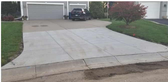
Figure 3. Example of additional concrete driveway replacement for curb stop repair where property owner paid or was assessed cost to replace additional area.
